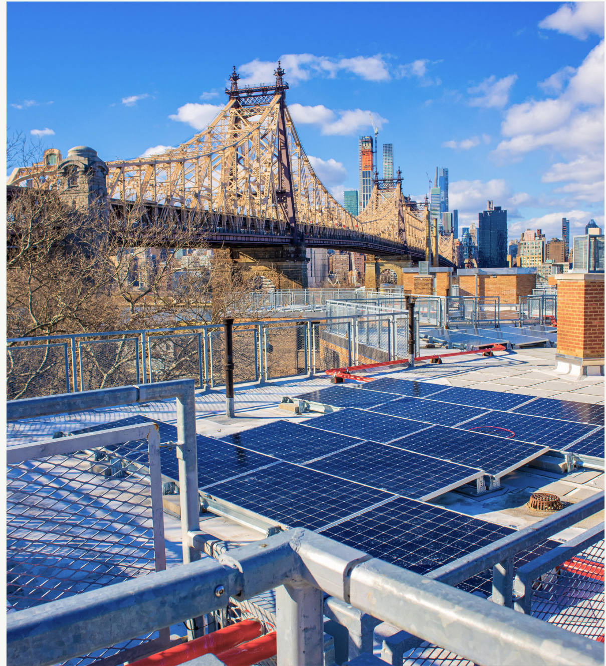
Solar panels installed by Sunwealth, an RSF borrower.
